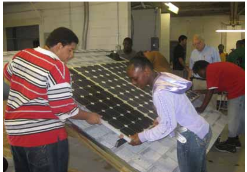
Supervised by program supporter Dr. Dave Edwards, students had the opportunity to experience solar panel installation.
